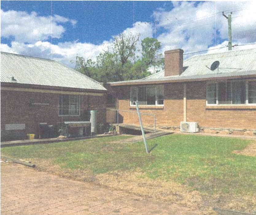
Rear view, indicating the lower roofed late 1960's addition on the left
