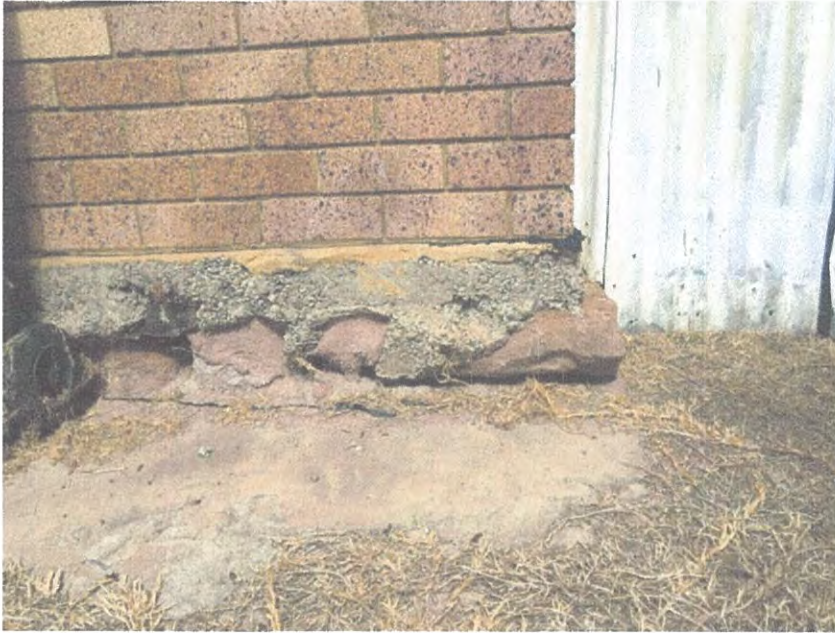
Base of wall at the rear, showing how the original stone perimeter wall has been used to retain the fill and support the concrete slab and cavity brickwork of the 1960's addition.
